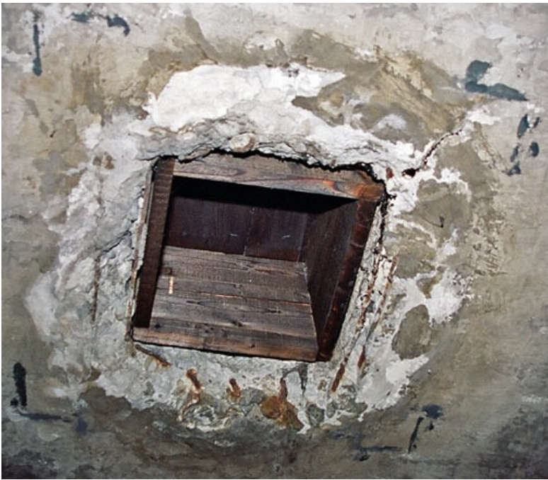
Crude holes put in by Russians, turning a morgue into a 'gas chamber'.
